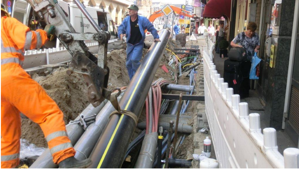
Figure 6: Picture of underground infrastructure in a city center.
